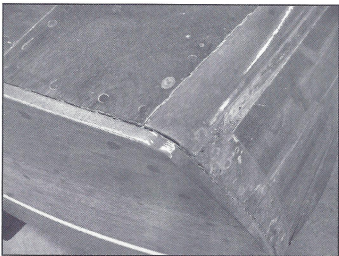
Transom planks pulling away from the sides.
